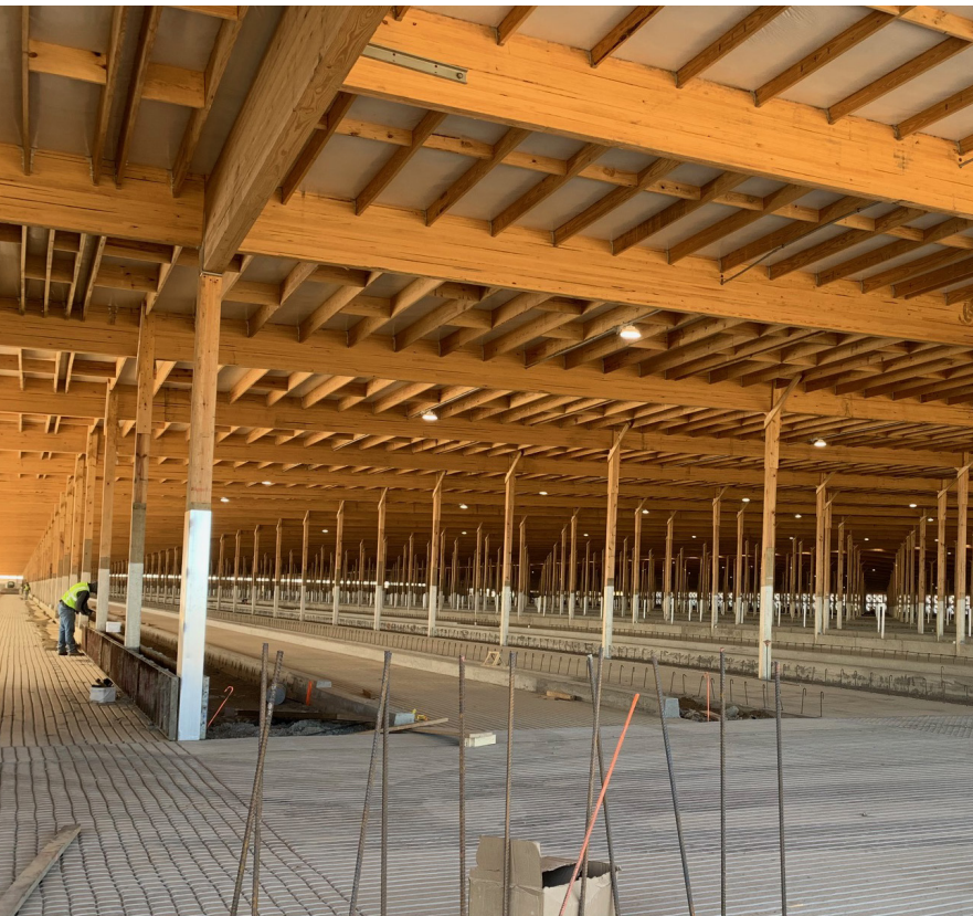
Construction of Garfield Dairy has taken more than a year and a half. The operation will include on-site employee housing and a 910,000-square-foot free stall barn.
